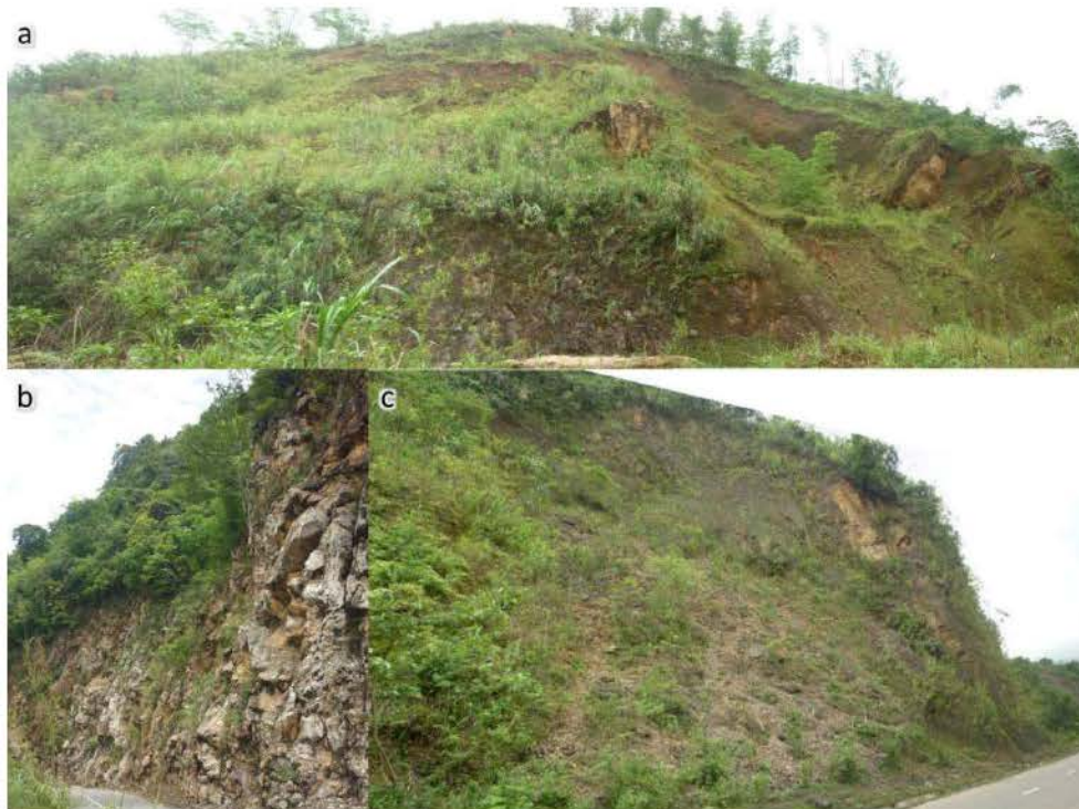
Figure 2.5 Some pictures of landslide along National Road No. 6 (photograph by Le): (a: landslide at Km 141+200; b: rockfall and topple at Km 128+700; c: rotational slide at Km 111+850).
