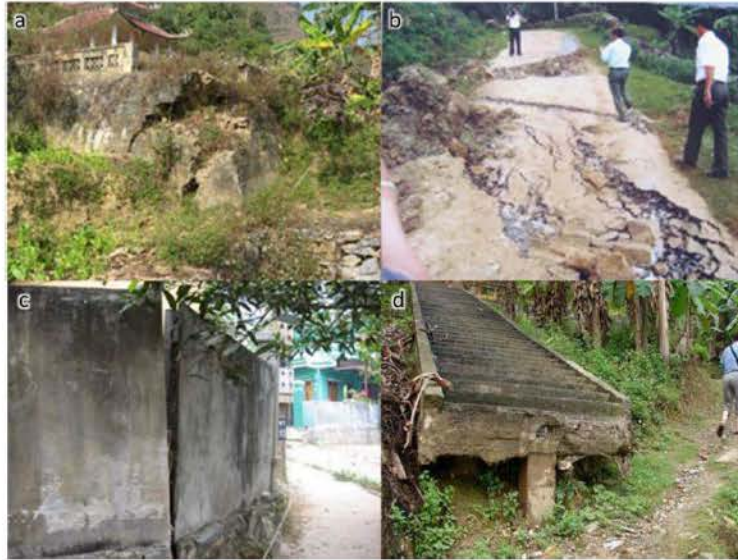
Figure 2.2 Landslide damage in Coc Pai downtown (Tran, 2009): a: landslide-damaged monument; b: boundary of landslide cuts throughout the road; c: house fence tilting because of landslide; and d: landslide movement of steps
