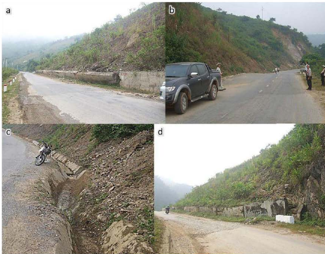
Figure 2.7 Images of landslides along National Road No. 7 (photograph by Le): a: retaining wall damaged by landslide; b: road was uplifted; c: ditch was bent; and d: landslide damage to a road and retaining wall
