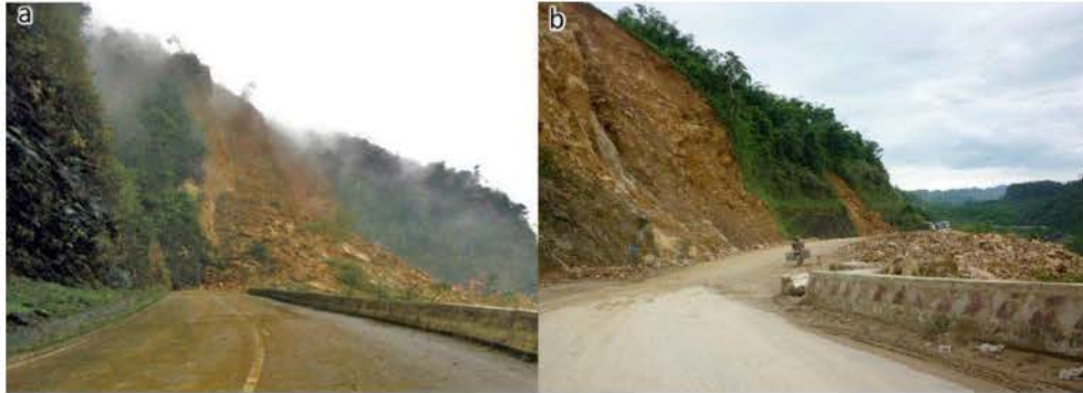
Figure 2.4 Landslide at Km 138+750 (a, Pham, 2014; b, photograph by Le): a: this picture was taken at the time the landslide occurred, 30,000 m 3 debris fell after a period of heavy precipitation and caused traffic congestion in 7 days; and b: was taken two weeks after landslide occurrence
